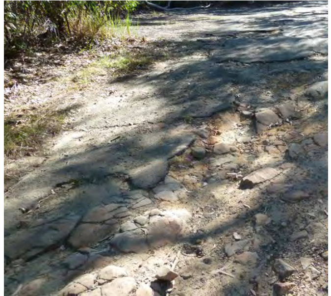
Plate 1.31: Erosion in the fire trail areas
