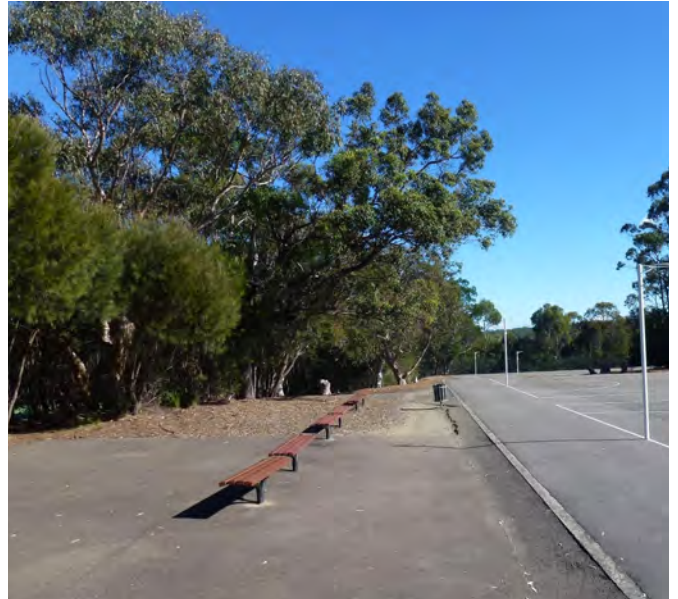
Plate 1.33: Eroded areas adjacent the path network
