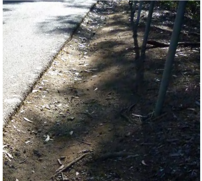
Plate 1.24: Erosion adjacent pathways/drainage swale
