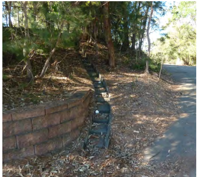
Plate 1.36: Open drainage system blocked with debris
