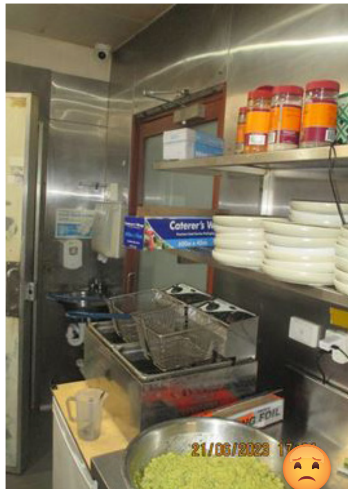
Example of deep frying without an approved commercial mechanical exhaust hood
